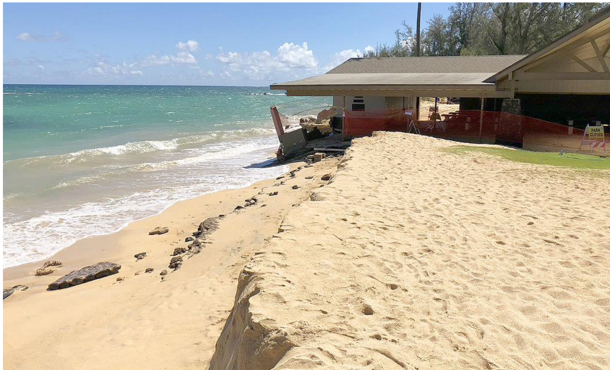
Figure 15: Damage to Baldwin Park Pavilion, August 2020
