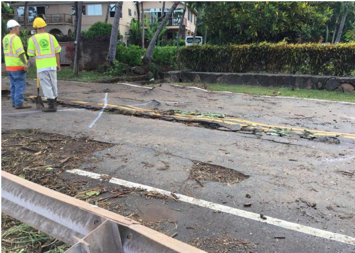
Figure 12: Damage to Lower Honoapi‘ilani Road, 2018
