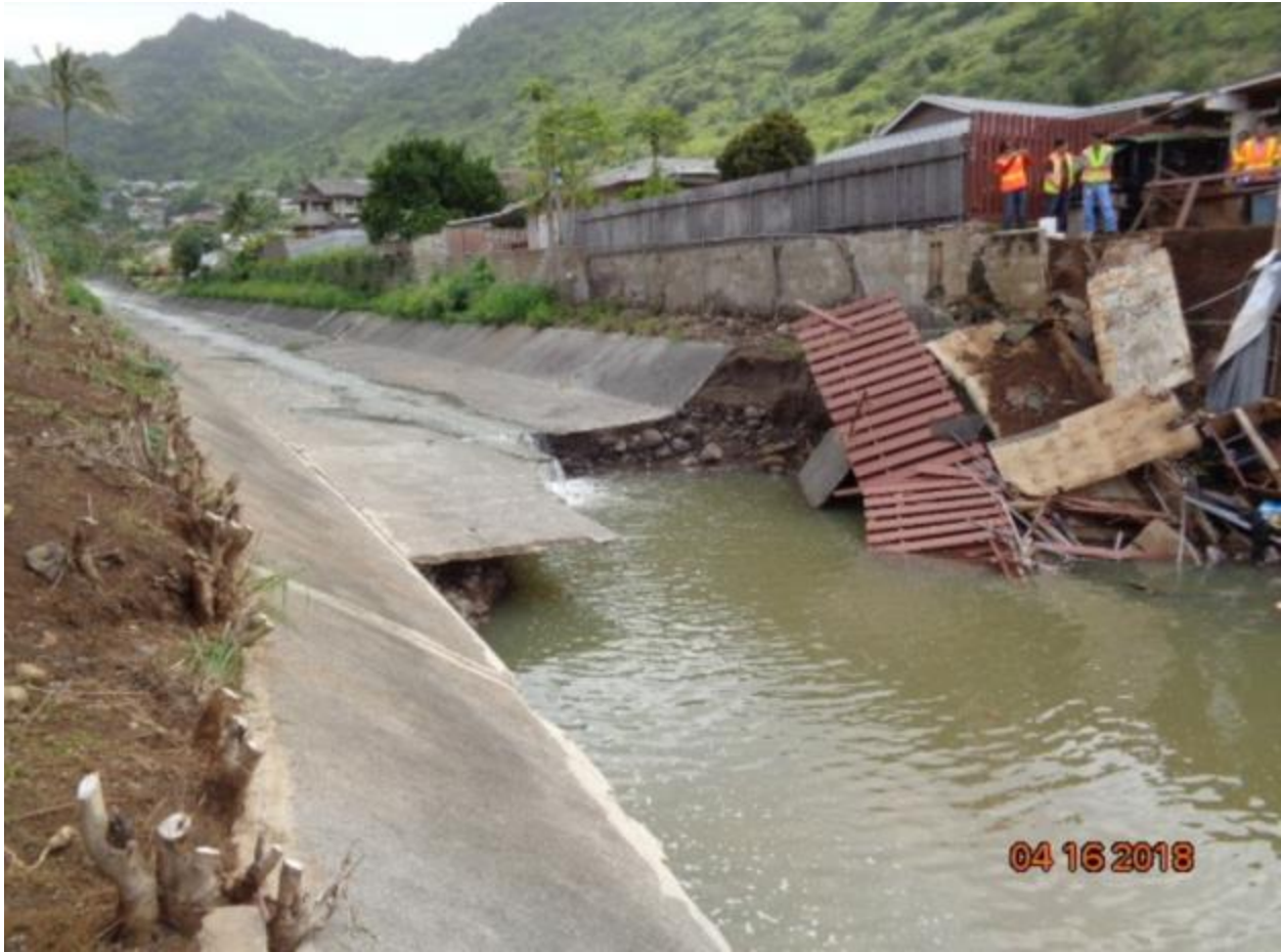
Figure 8: Destruction of the Hahaione Channel After Rainbomb Event, 2018
